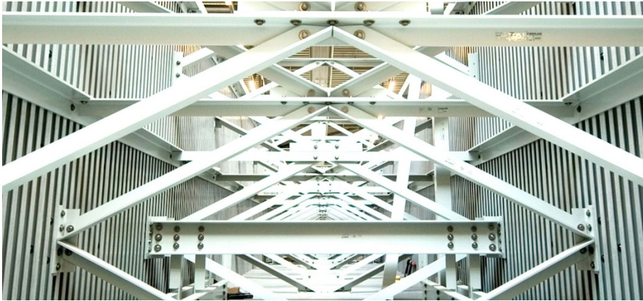
Figure 1.2 - Application of pultruded FRP angle section profiles as lateral bracing (Source: fiberline.com/design-manual , accessed on Feb 20, 2024).
