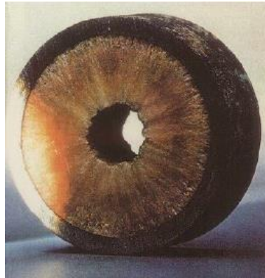
Figure 1 – Wax deposit reducing the effective diameter in a retrieved pipeline (Singh et al., 2000).
