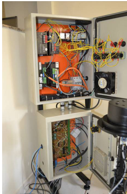
Figure 5.1: Electrical peripheral system.
